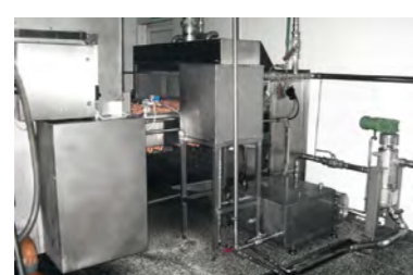
Liquid smoke unit with showers in circulating tank and storage tank as well as rotation filters and pumps.
